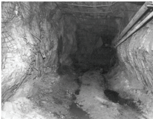
(a) Yielding ground conditions
