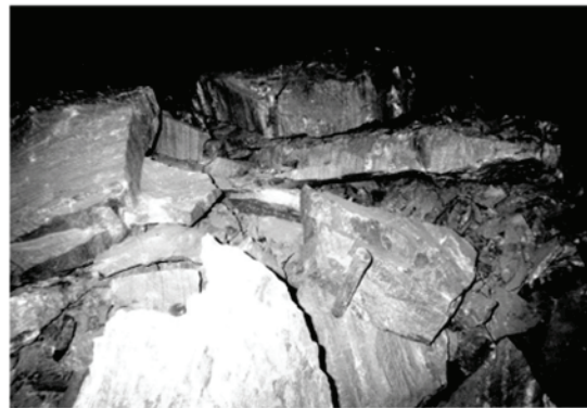
(b) Catastrophic failure of back and rock bolts
