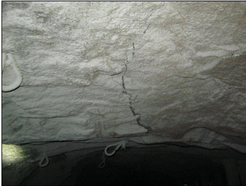
Figure 9: Open fracture in the ASG hangingwall
