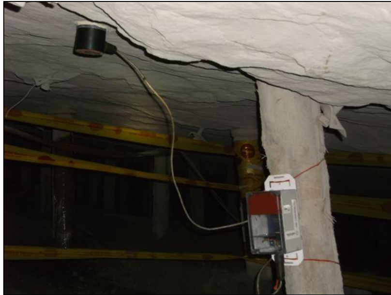
Figure 11: Installed FOGWarn unit
