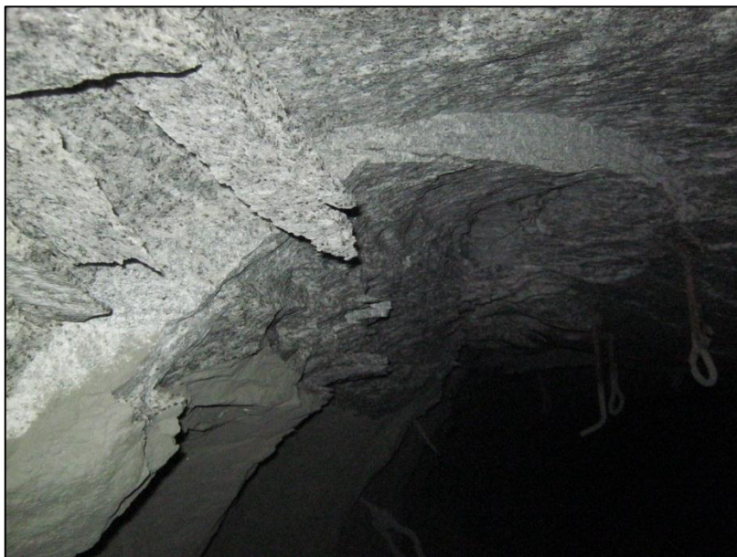
Figure 8: Scaling at the pillar/ASG interface
