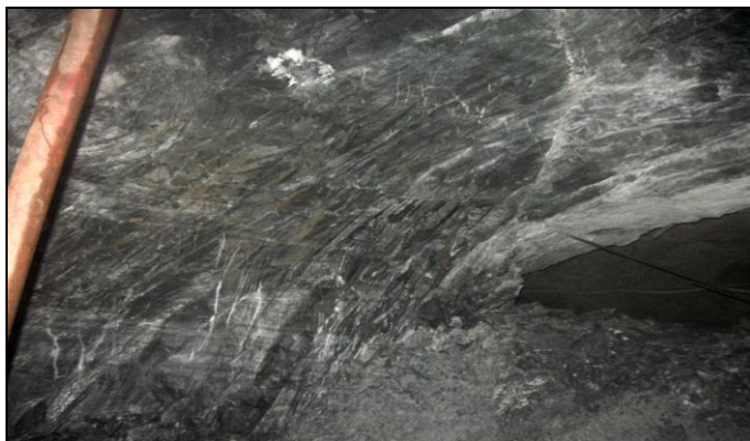
Figure 16: The highly stressed toe of a panel where leads and lags were out of standard.
