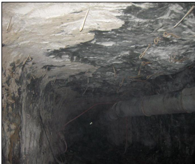
Figure 18: Stress related hangingwall scaling in a north-west orientated tunnel.
