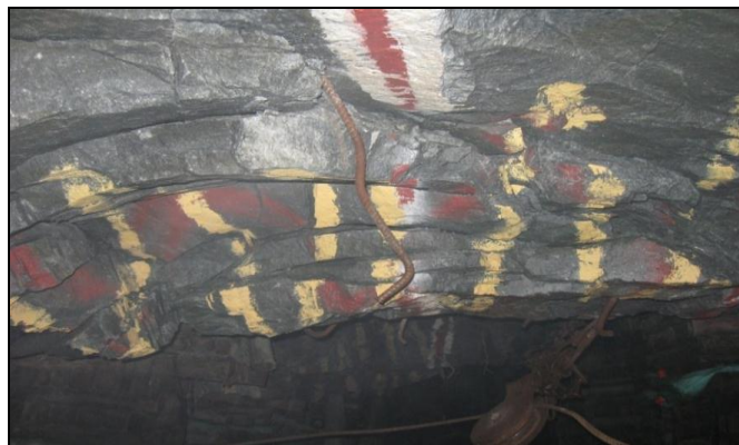
Figure 14: Stress fracturing above a gully.
