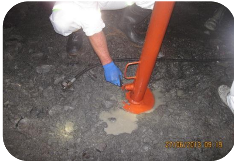
Filler pistol connected to filler valve
