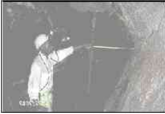
Figure 1. Picture showing ground damage after the occurrence of a seismic event
