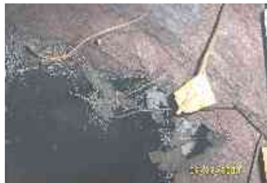
Figure 5. Picture showing ripped diamond mesh and protruding roof bolts after a seismic event
