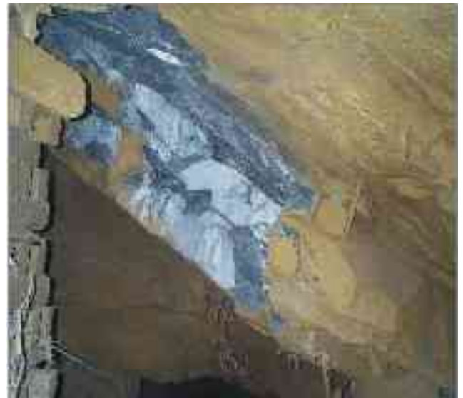
Photo 6: Rockburst damage caused to a brow in the W1 gully.
