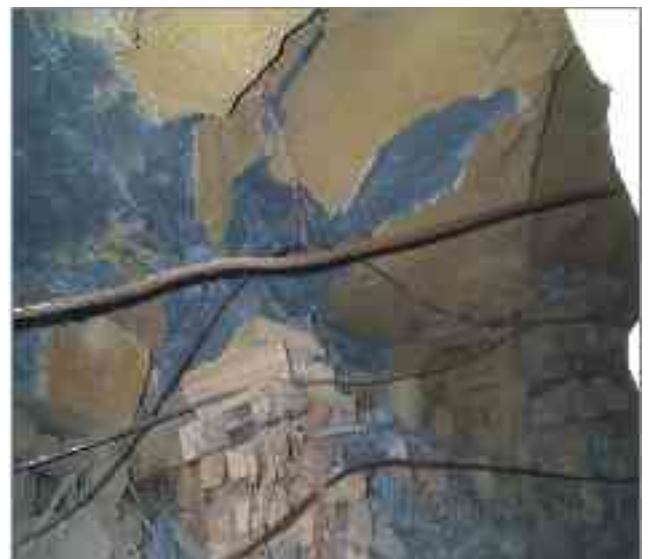
Photo 7: Rockburst damage caused to hangingwall of the W1 gully next to a strike stabilizing pillar.
