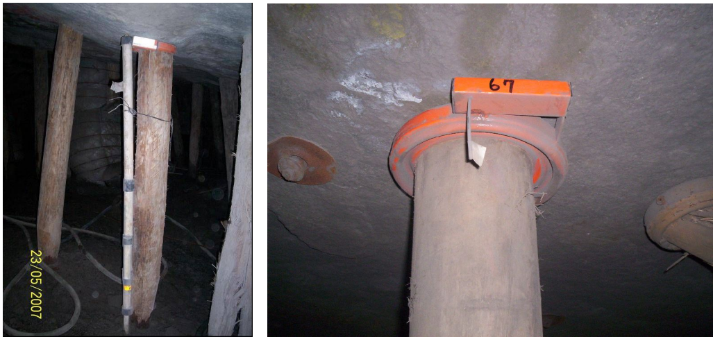
Figure 11. Closure and Load Loggers installed with a pencil prop in a deeper platinum mine
