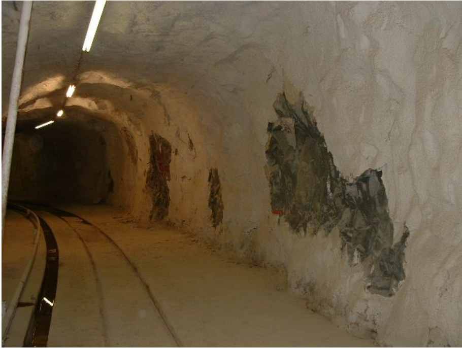
Figure 7. Haulage sidewall scaling in the shaft pillar area.
