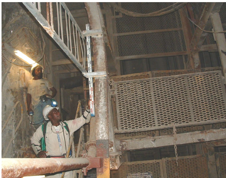
Figure 6. Significant bending of the kingposts on 33 level station. This area has been subjected to compression, possibly due to a previous episode.
