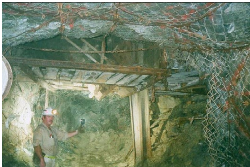
Figure 89: Sidewall ejection after pillar failure (left) and complete collapse of a tunnel as a result of seismic energy release
