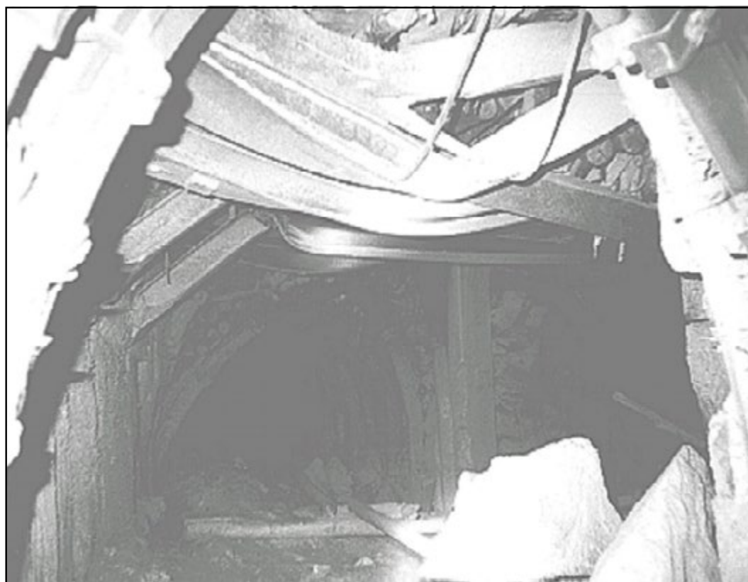
Figure 15: Steel arches in drawpoints (Courtesy of Petra Diamonds)
