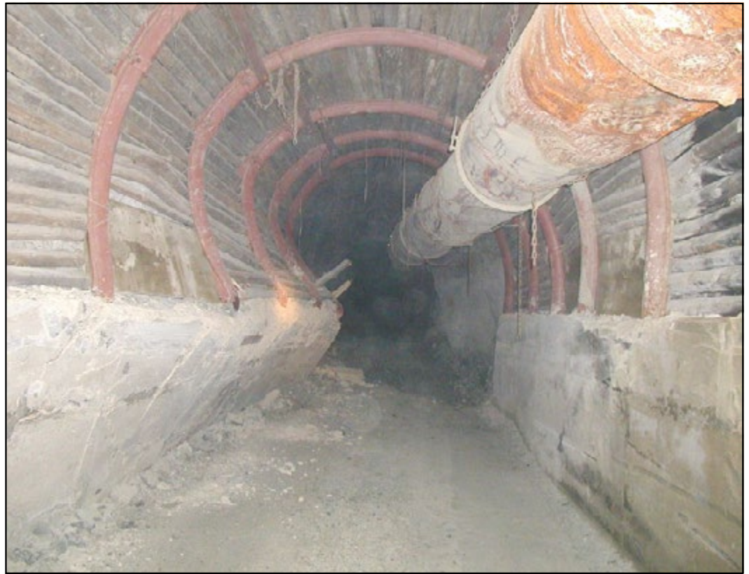
Figure 17: Steel arches and timber lagging in drawpoints (Courtesy of Petra Diamonds)
