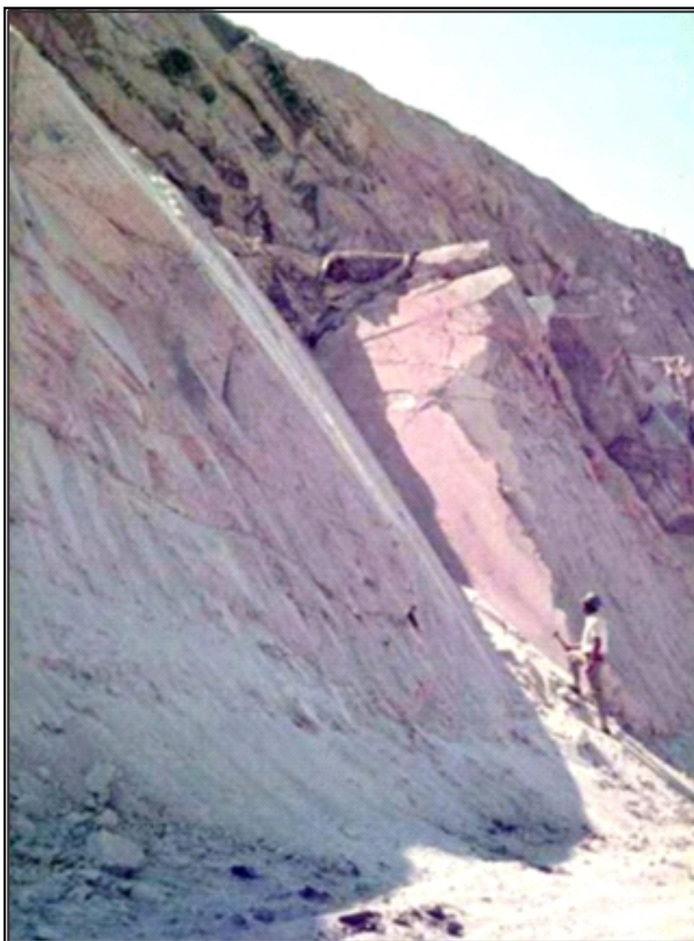
Figure 9: A typical example of wedge failure in a slope face (Hoek, 2007)
