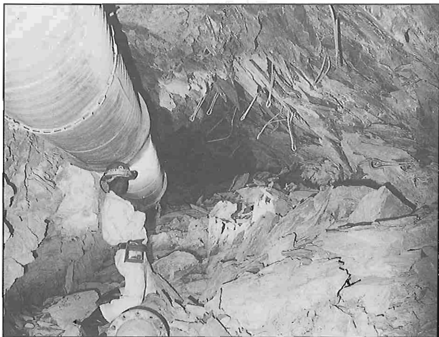
Figure 8.3.6 Damage to 34K footwall drive at Site A showing falls of ground between grouted shepherd's crook tendons. Mesh and lacing had not yet been installed in this section of the tunnel. In this area, the south-western (right hand) side of the drive was most severely damaged.
