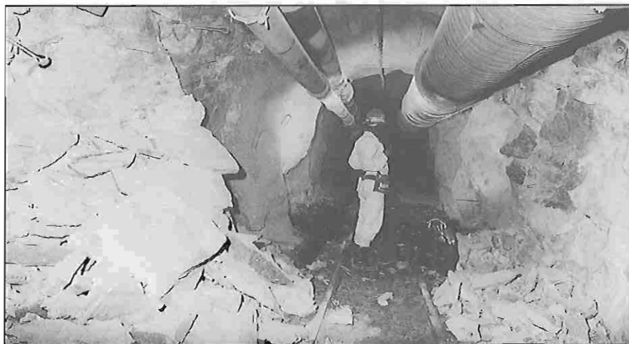
Figure 8.3.8 A haulage on 34 level showing the effect of the support system on damage. The section of the tunnel in the foreground was supported only by grouted rebars, and significant damage was sustained. The support system in the section of the tunnel beyond the miner consisted of grouted rebars, mesh, lacing and shotcrete. Damage was negligible.
