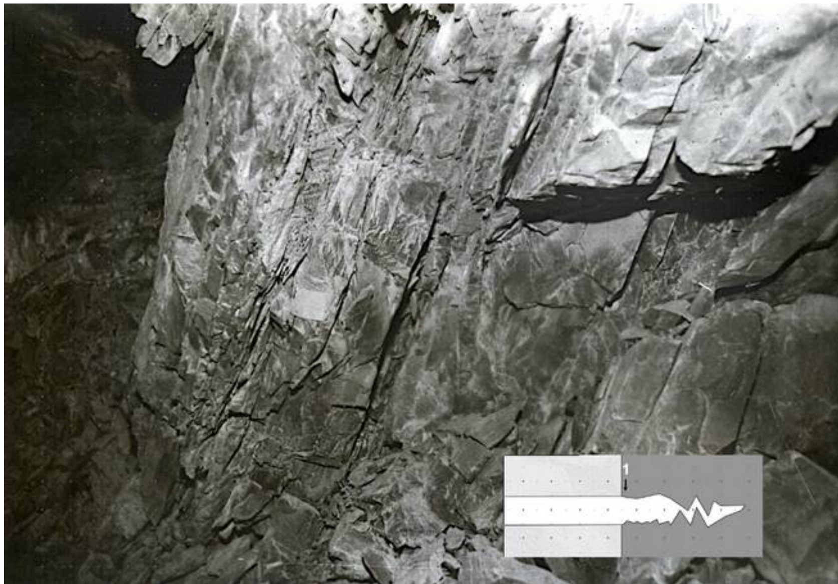
Figure 9: Fractures at position 1 in the section shown in Figure 8
