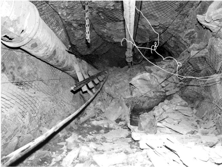
Damage to an access tunnel
