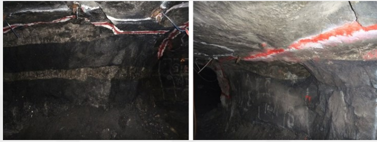
Figure 2: Pillar-forming material at Booysendal South Mine.
