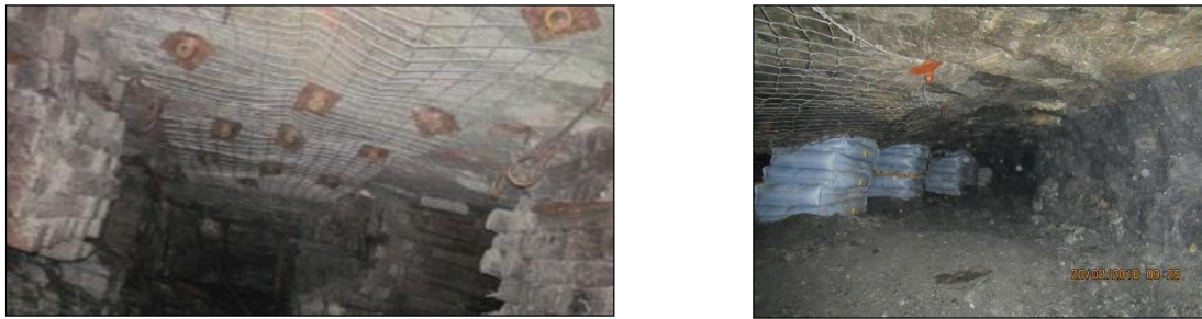
Figure 1. Welded mesh installed in a deep gold mine gully (left) and permanent blast resistant chain-link mesh installed in-stope on a narrow tabular platinum stope face (right)
