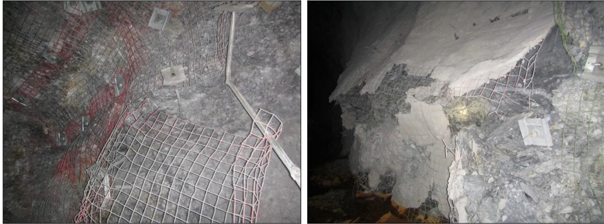
Figure 14. Poor faceplate contact resulting in the failure of the mesh strands as it loaded laterally against the rockbolt
