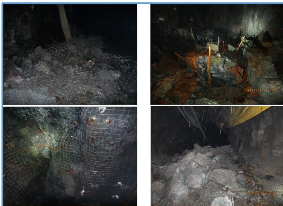
Figure 2: Typical falls of ground in the rooms
