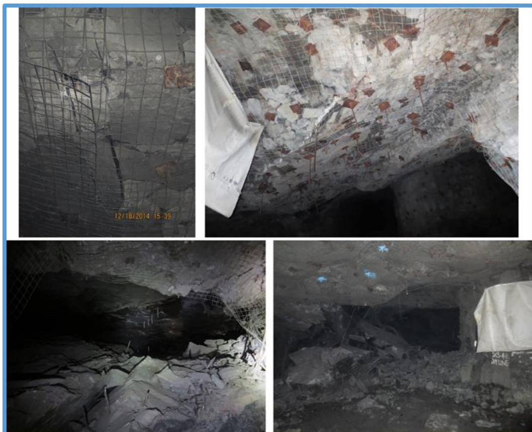
Figure 4: Deformation of room hangingwall
